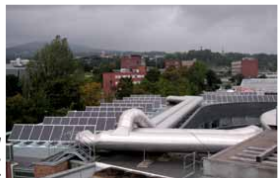
Grid connected system, Oslo Innovation Centre
